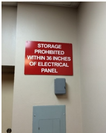
Obstruction of Electrical Panels
