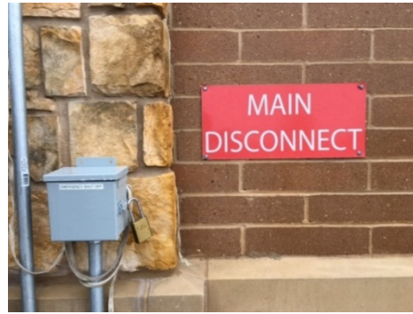
Utility Disconnect Signs
