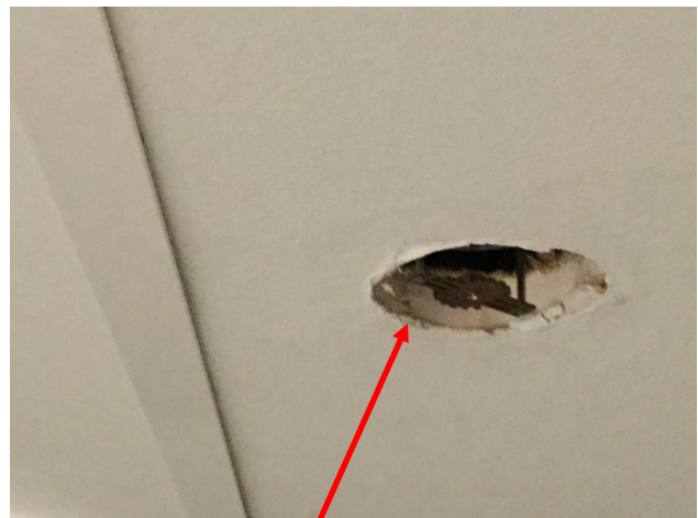
Concealed head with no clearance below the ceiling surface
