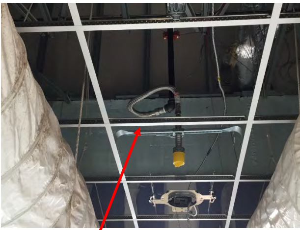
Failing to maintain the 4" minimum radius & number of bends allowed for 2' hose in violation of the U. L. Listing
